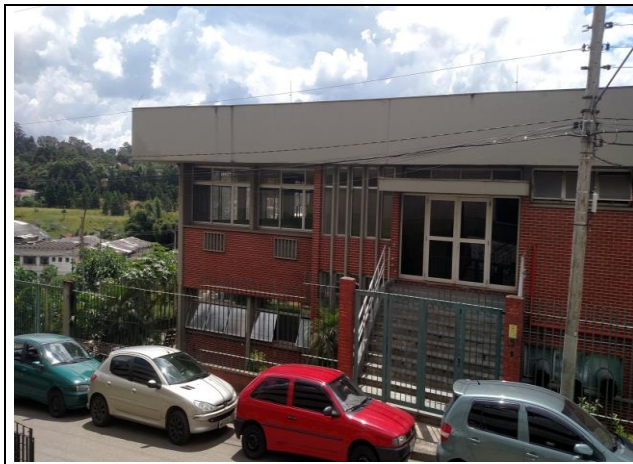
Porta Fachada principal avariada
